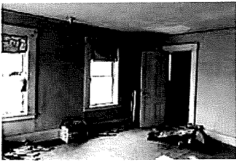
The interior of this 19th worker's house has not been properly maintained, but it may be as important historically as a richly ornamented interior. Its wide baseboards, flat window trim, and four-panel door should be carefully preserved in a rehabilitation project. Photo: NPS files.
