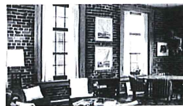
Plaster has been removed from perimeter walls, leaving brick exposed. The plaster should have been retained and repaired, as necessary. Photo: NPS files.
